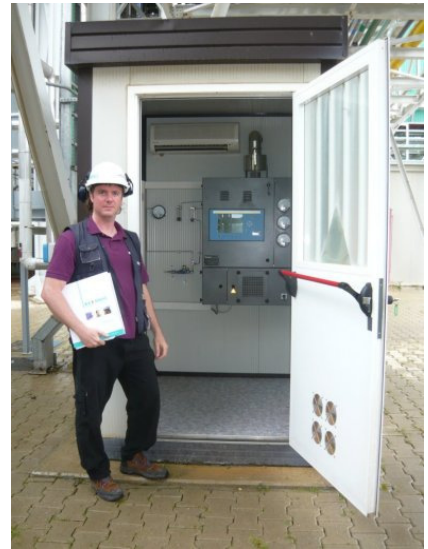
Maintenance in Italy (Shelter Design)
